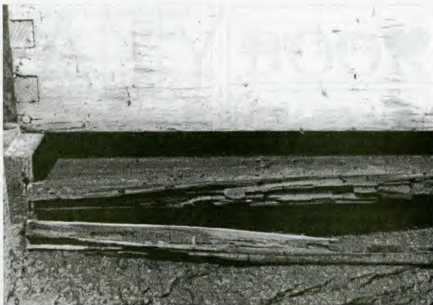
Replace equipment that's been 'weathered' immediately, and check the rest.
