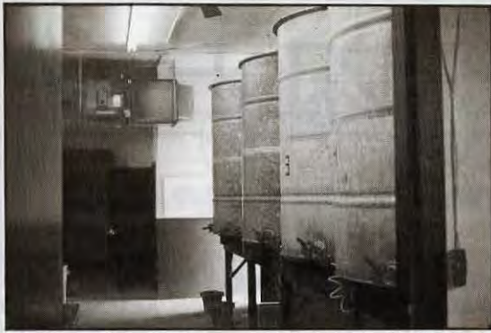
The four 700-gallon galvanized holding tanks. When one is full all 13 barrels are considered a 'lot'.
