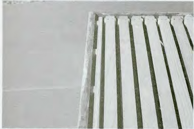
Note the space between the spacer board and the adjacent frame.
